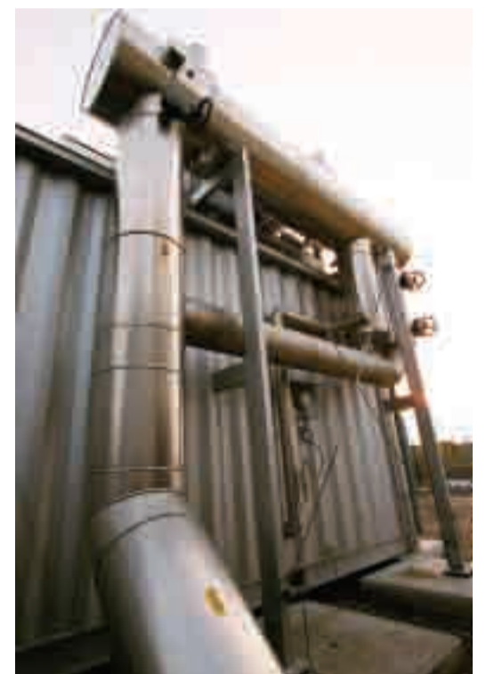
CIAT tubular heat exchanger system at the entry to the gas preparation container (installation with Bypass and condensate separator).
