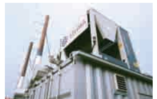
AQUACIAT 2 installed on the SILOXA gas treatment container
