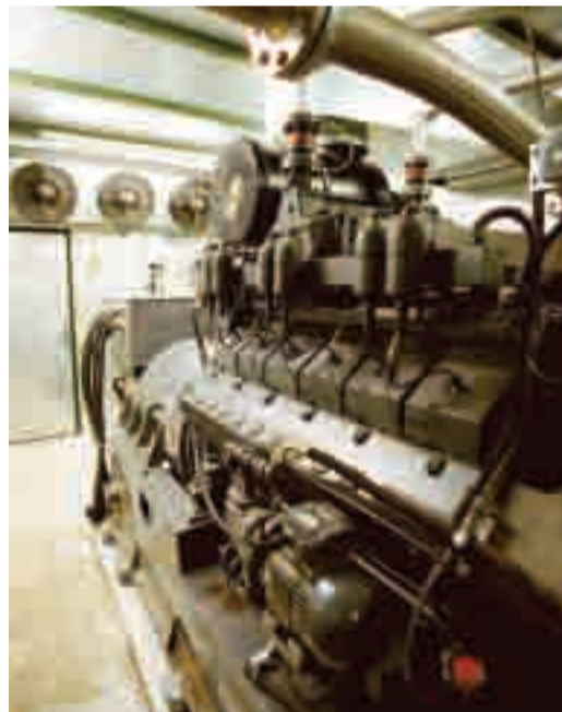
Containerized gas engine
