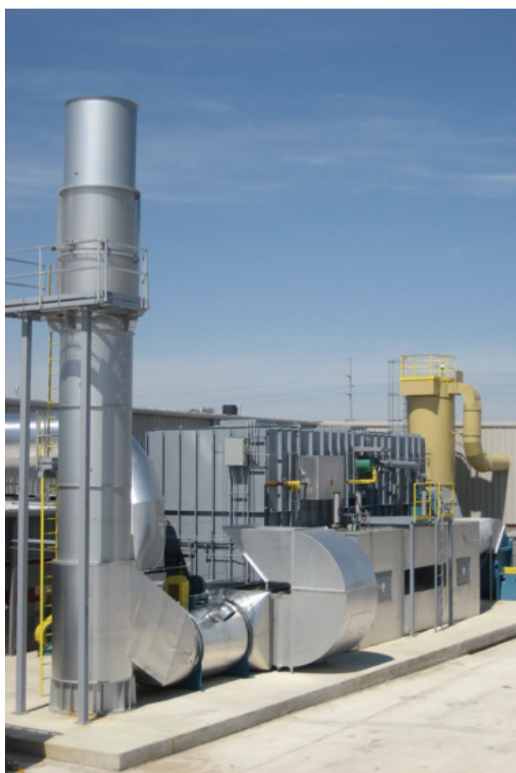
A Regenerative Thermal Oxidiser (RTO) with secondary air-to-air heat recovery system that is using recovered energy to heat process cure ovens.
