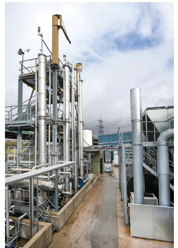
UKCCSRC PACT carbon capture plant
