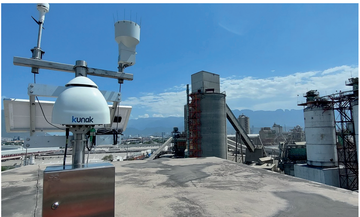
Kunak AIR Pro station installed at CEMEX Plant in Monterrey (Mexico).
