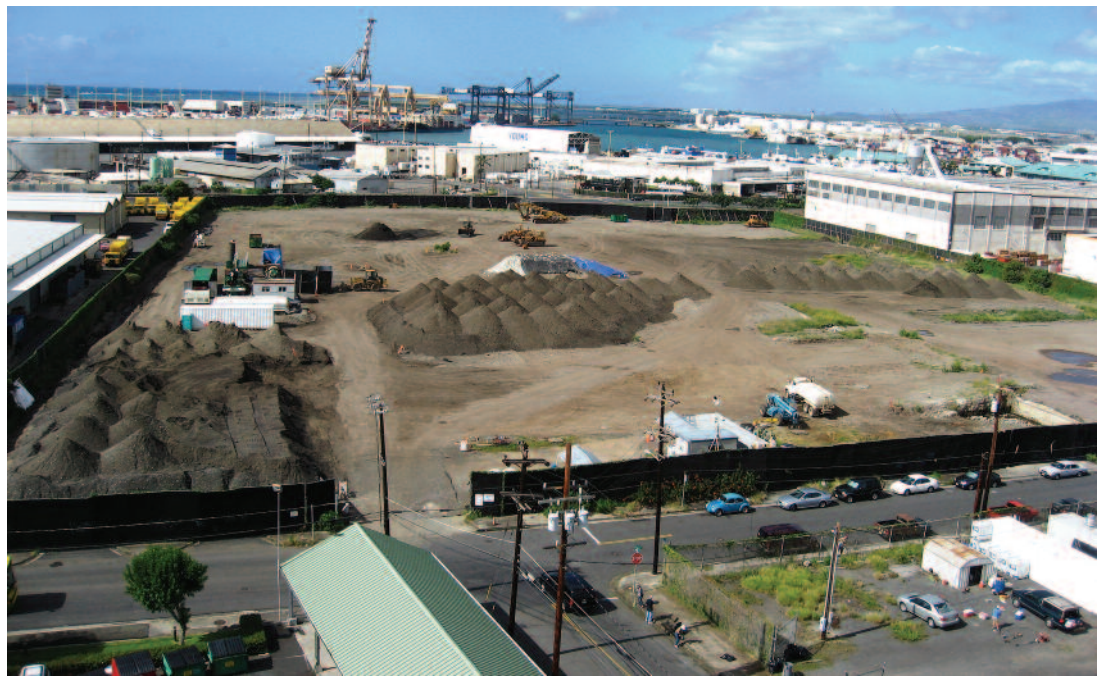
Fig 1. Creating Clean Dirt, No Doubt! at a refinery soil remediation project, Honolulu, Hawaii
