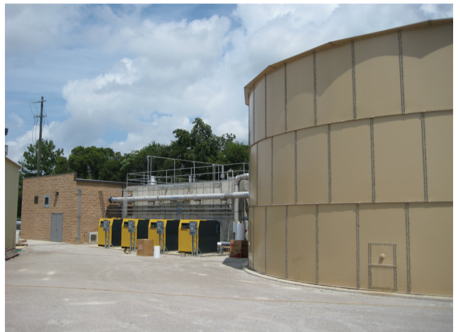
ADI-MBR system at Golden Flake, showing the pre-aeration tank (right), pre-cast concentrate membrane tanks and aeration blowers (center), and operations building (left). The operations building houses the electrical systems, PLCs, sludge dewatering system, pumping systems, laboratory and office. The entire footprint of the MBR system including the operations building is 140 ft. by 60 ft and treats 400,000 gpd of raw wastewater.
