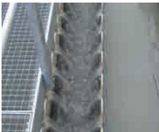
fig. 2: clean water weir in the Leiblein lamella separator
