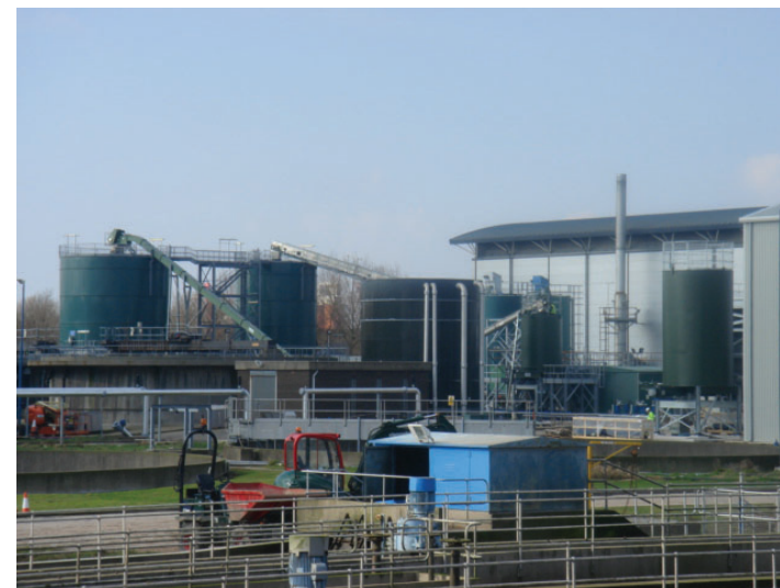
Saxlund Sludge cake handling system
