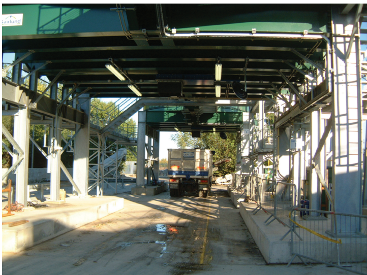
Truck loading Saxlund system for waste water
