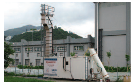
ANAMMOX® pilot plant for on-site testing
