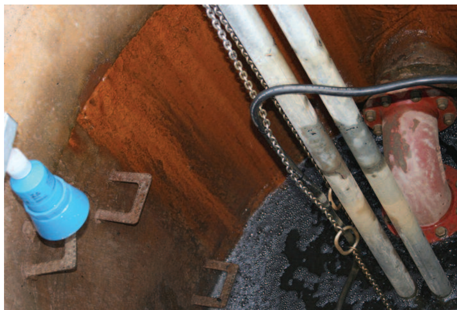
Siemens Echomax transducers installed in the well and the Sitrans LUT400 controller measure the level of water and control pump operations.
