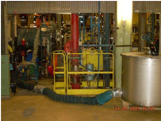
Vapour extraction and active carbon filtration
